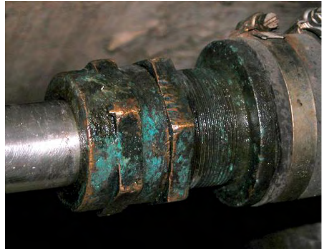
Check shaft inside boat, shaft log and stuffing box. Replace stuffing if needed.
