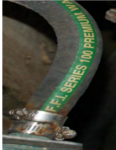
Check hoses and hose clamps. The bottom one could use replacement.
